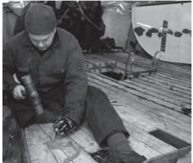
Caulking of decks is an important skill in the upkeep of the old vessels. Maintenance using traditional techniques and materials is important for retaining the historic value of the vessels.
