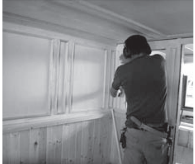
Interior works on a fiord steamer, a steel ship. Bredalsholmen, one of the ship preservation centres, has the expertise for steelwork. The other two centres' expertise is with wooden vessels. Hardanger Fartøyvernssenter carries out interior work on steel ships.
