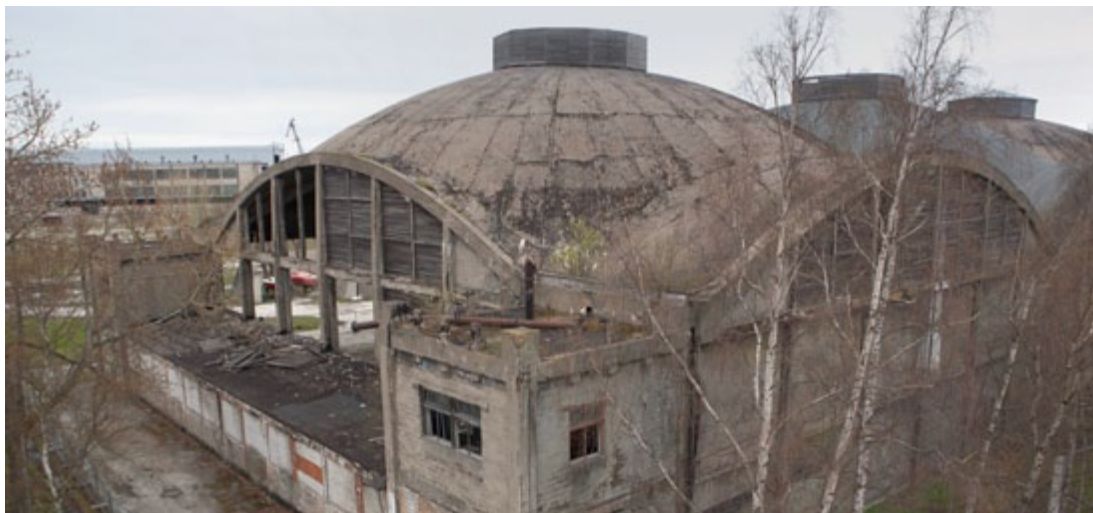
The hangar shells were in terrible condition, very near to collapsing / 2009.
