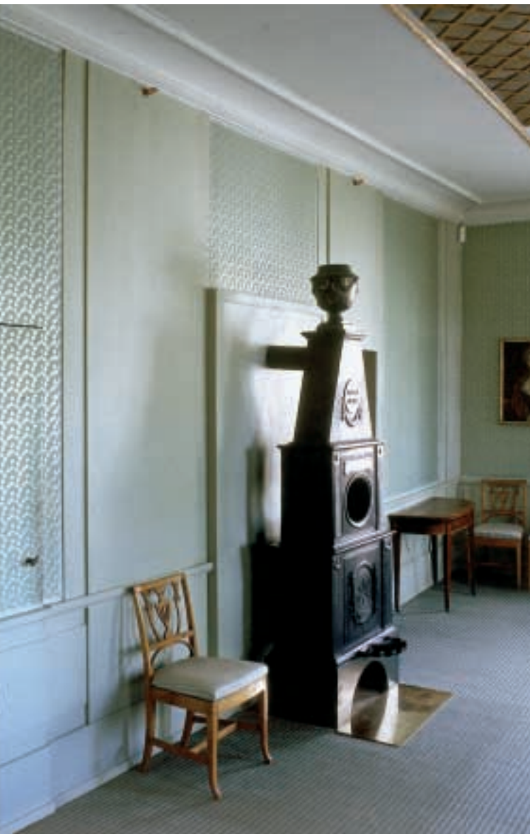
Sprinkler heads do not disturb the space very much if installed carefully.
