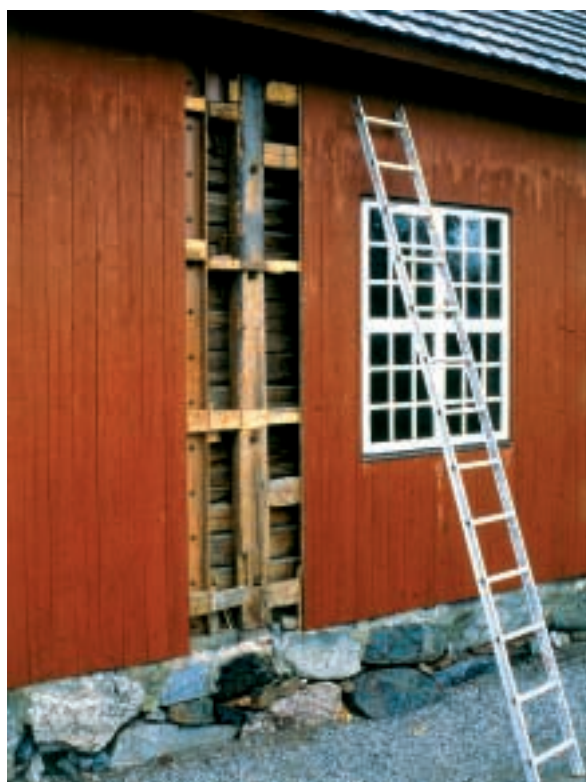
The gap between the log wall and the exterior boarding.
