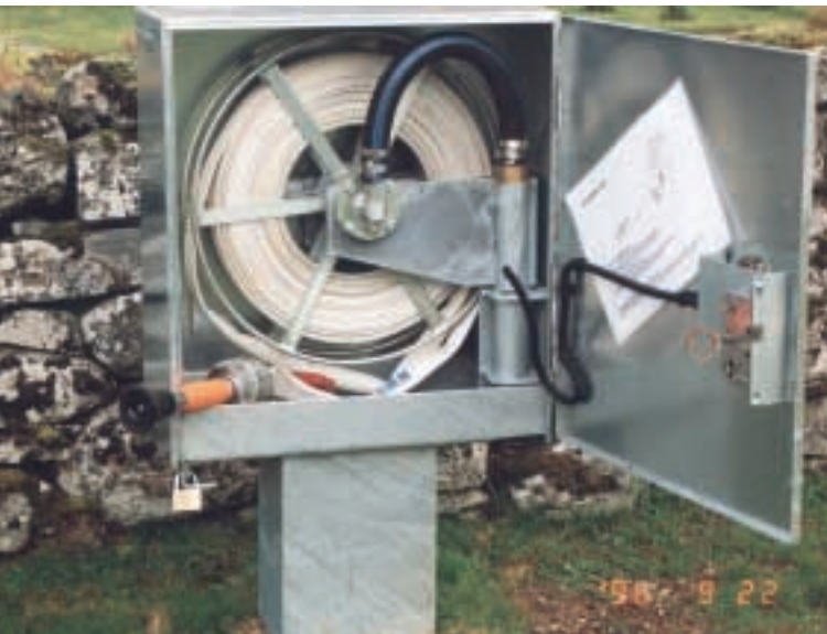
Fire hose boxes should be designed to match the surroundings.
