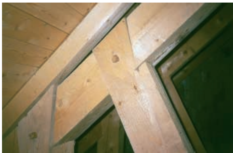
Detail of the new roof construction made of timber with wooden joints.
