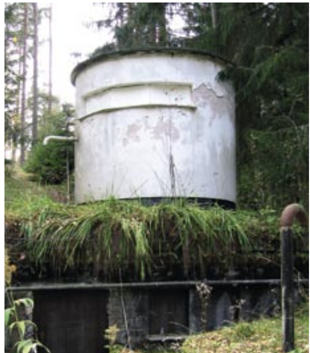
Fig. 16. The water pumping station.
