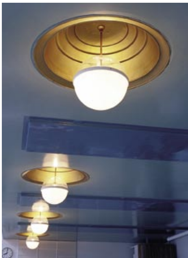
Fig. 17. Dining hall lamps and radiant heaters in the ceiling.
